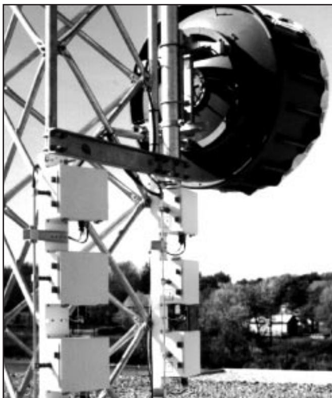
Multiple MR-23CX RF Units with 4' Antenna.
